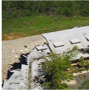
The Lake Guntersville State Park Lodge in Alabama was destroyed during tornadoes. The damage caused District 6860 to cancel its annual conference.
